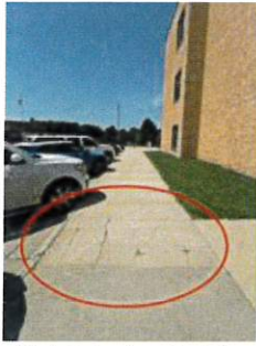
High School south side. Recommend replacement of damaged concrete to prevent possible trip and falls
